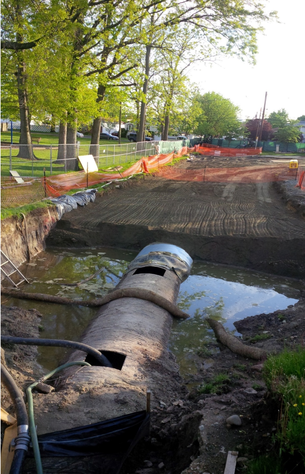
Fig. 3. Redstone Park storm pipe bypass pumping operation during Phase 1 (note: trees on left were removed during Phase 2 to allow for excavation).
